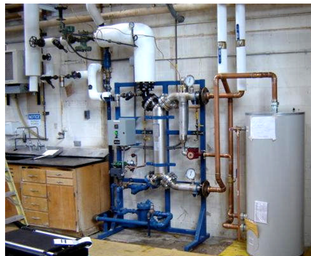
Duplex 65 gpm Domestic on 125 psi steam
