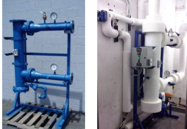
250 gpm Building Heat on 60 psi steam
