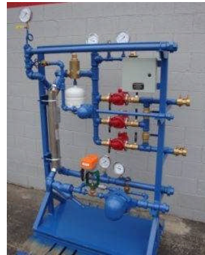
Multi-zone Building Heat on 40 psi steam
