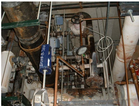
Fig 7 Complicated steam and drainage piping
