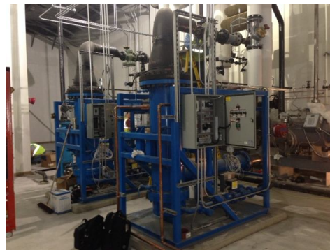
Fig 8 Advanced Steam Technology XE Thermal Skids
